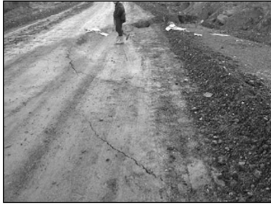
Figure 2. Shearing occurred in the road due to slope instability. This road is at the Northeast border of the pit and around 150 meters away from Gumuspınar village houses.
