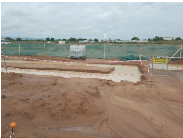
Figure 15. Caution tape and signs used
