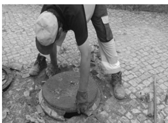
Figure 3 - Lifting the lid of the collector.
