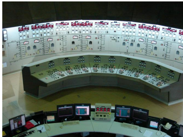
Figure 1. The Typical Room of the Electric Power Control Center
