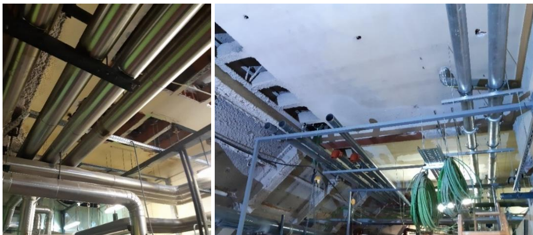
Figure 3: Real cases with MEP supports defined on the jobsite.
