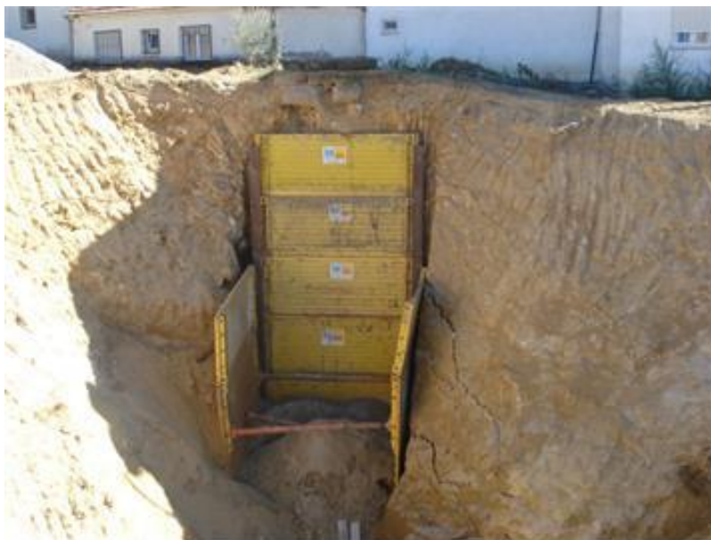
Figure 3. Berlin retainer used on site (Henrique, 2017).
